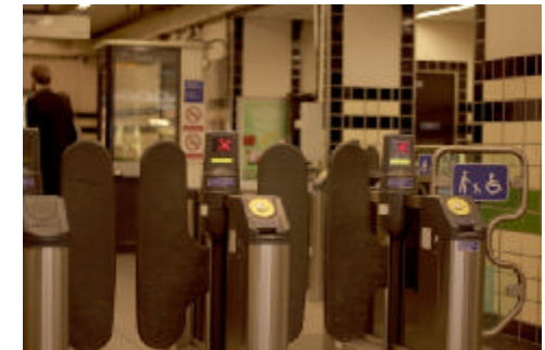
Automatic ticket gate
